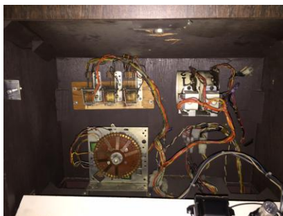
Upper cabinet wiring
