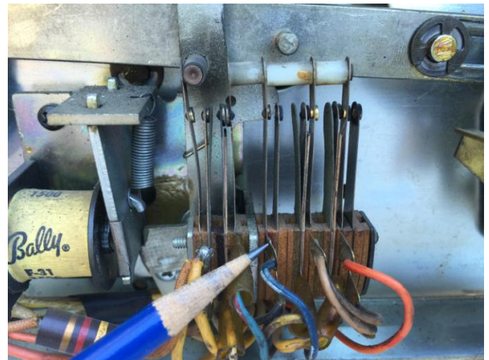
Some [of many] reel assembly relays
